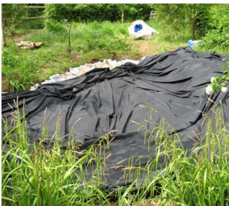
Laying pond liner for a new pond. See A64 for step by step construction.
