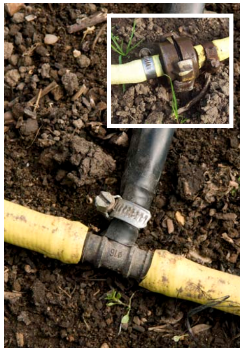
Hose connections. Similar drip pipes are available for individual plants. Clean these regularly.
